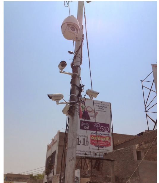
Cameras at intersection location
